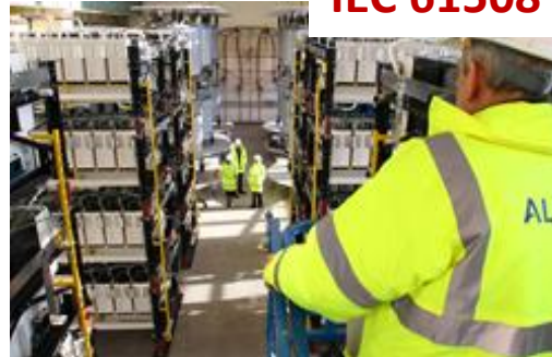
GE Power HDVC Power Systems
